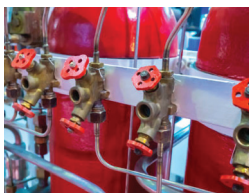
Foam & Chemical Systems
