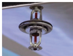
Wet/Dry Automatic Sprinklers
