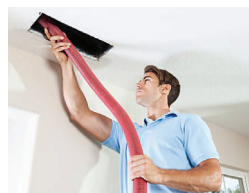
Hood & Duct Cleaning
