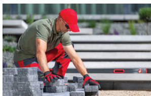
Roof Top or Terrace Gardens
